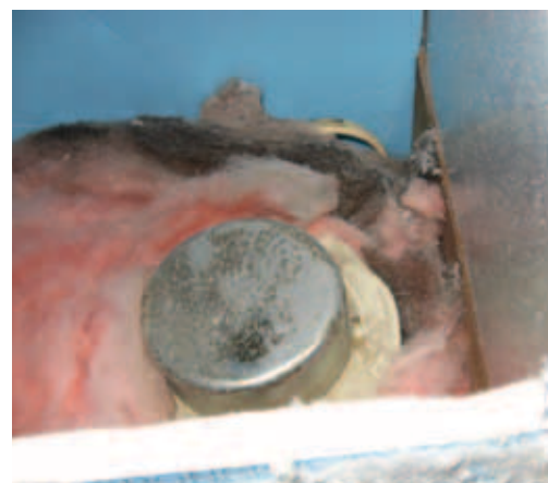
Fiberglass insulation is shown around an unsealed, dammed recessed light.
