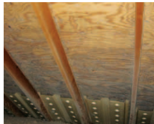
This photo shows the frost and evidence of the mold on the roof deck.
